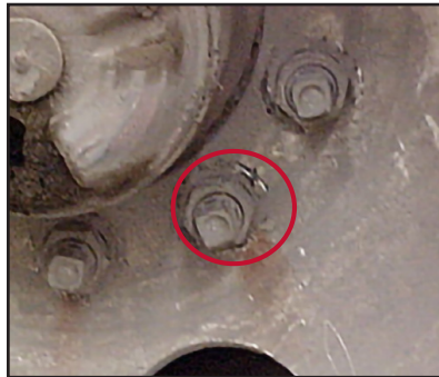
Bolt hole crack
