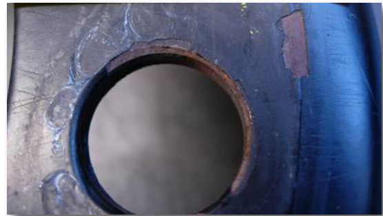
Shell with paint blistering in the leaking area
