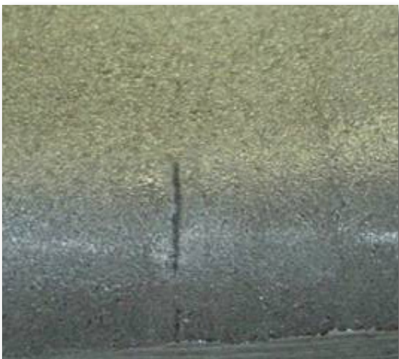
Crack in the rim welding seam
