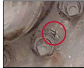
Bolt hole crack
